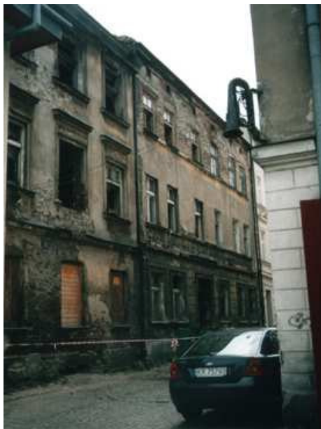
PHOTO 3. The corner of Izaaka and Kupa streets with extremely dilapidated, abandoned tenement houses seen on the left
